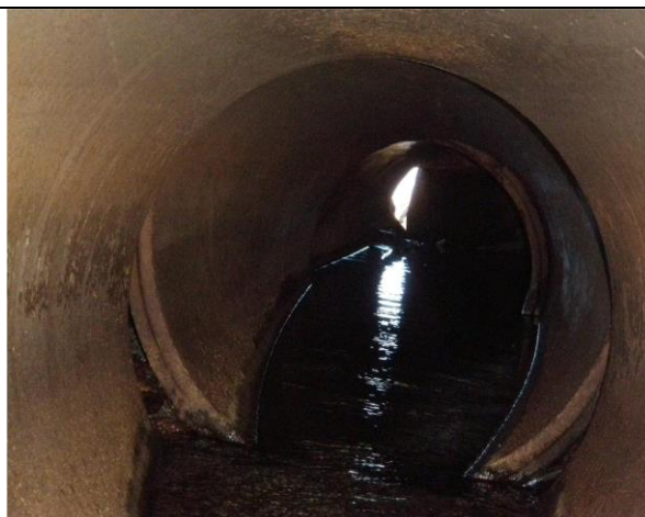
Photo inside pipe showing displacement
