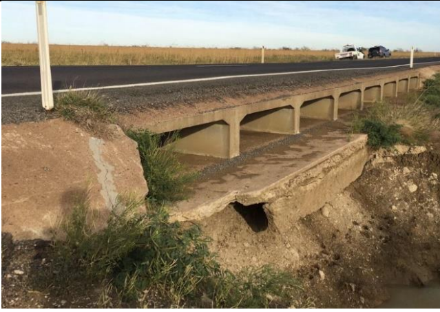
Post event photo of road and culverts undermined by the event
