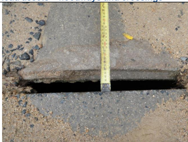
Tape demonstrating displacement of pipe
