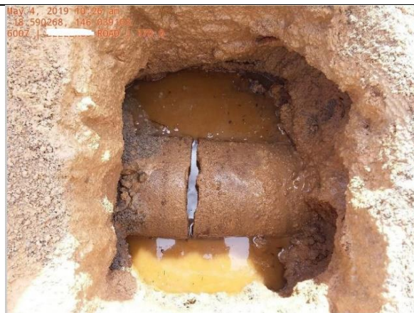
Detail of displaced pipe during investigation
