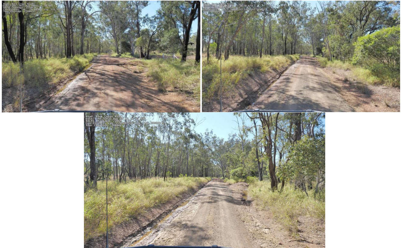
Above examples consistently spaced photographs along the asset demonstrating event damage
