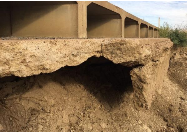
Close up of scour
