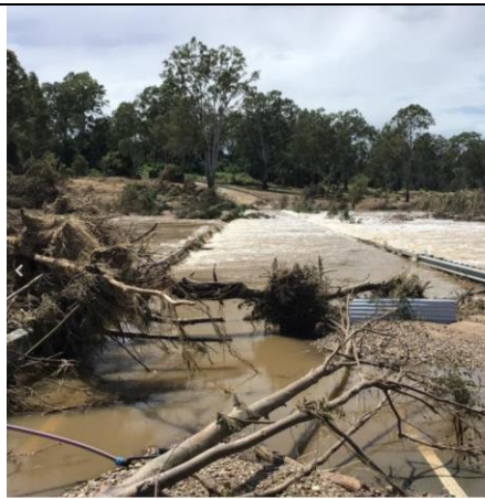
Geotagged photos taken after waters receded supporting the event impact on the asset and the need for the completed clean up emergency works
