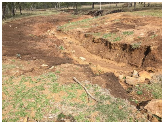
6. Rock protection displaced downstream.
