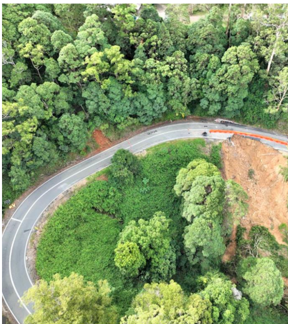
Above Landslip 2 – Drone view showing context and scale
