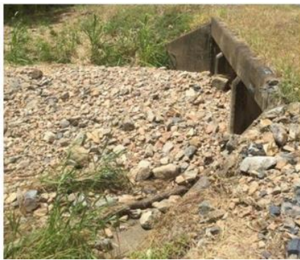
Side view extent of rock deposited against the culverts
