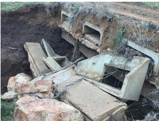
5. Closer view showing undermining and damaged components.
