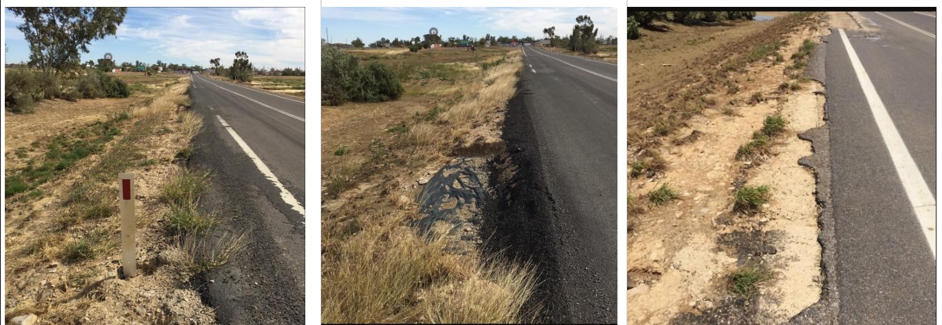
Above - examples of photos at regular intervals in the same direction along asset to support the extent of the event shoulder scour and scope of works
