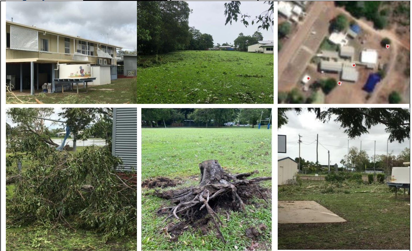
Above – State education infrastructure - Post event geotagged photos demonstrating the location and need for emergency works to remove event related debris impacting on school infrastructure. Clean up costs not covered by insurance may be claimed under DRFA.
