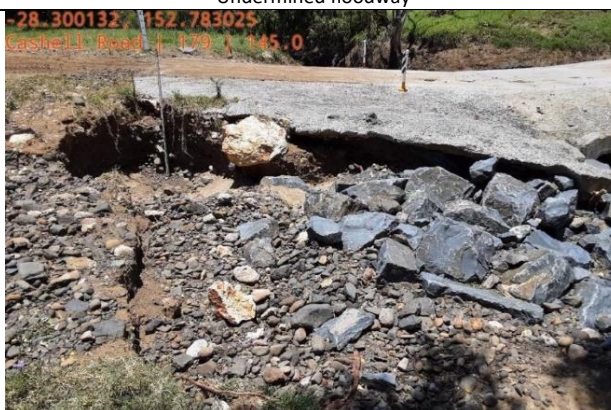
Side view further demonstrating extent of undermining`
