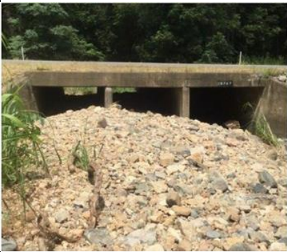
Post event photo downstream view of rock built up against culverts
