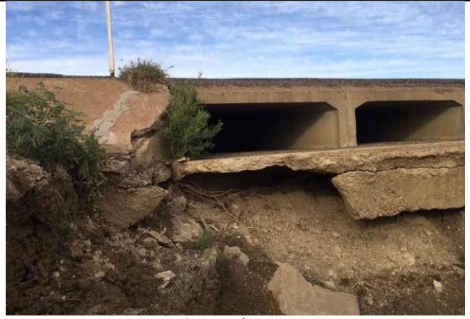
Side view of scouring
