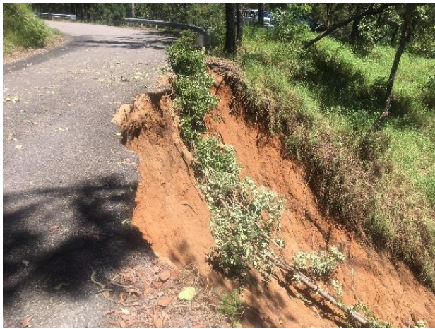
Landslip 1 – post event downside slip along asset
