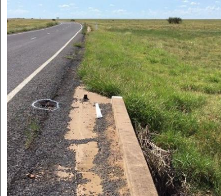
Mark-up identifying the damage site within the asset context
