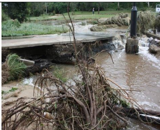
Undermined displaced floodway
