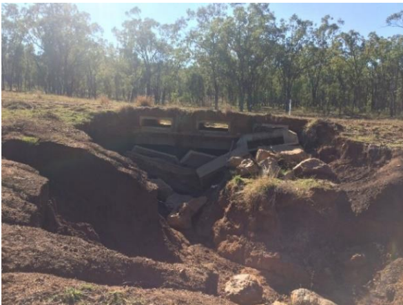
3. Upstream view of the extent of event damage to the asset components.
