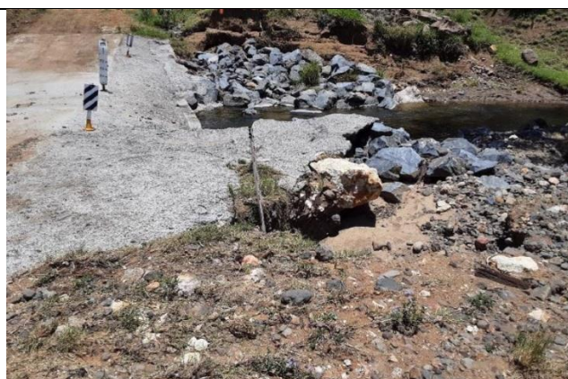
Approaching undermined floodway
