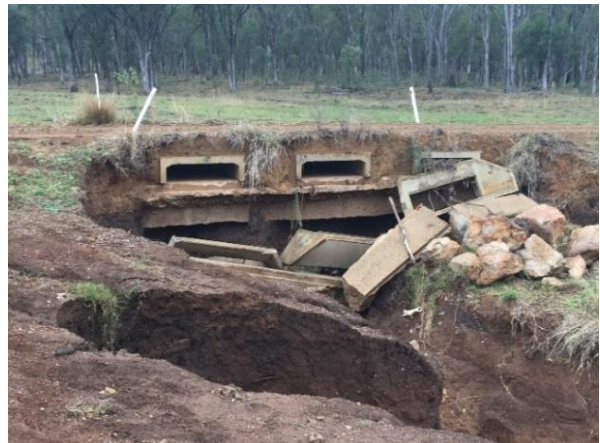
4. Closer upstream view of damaged components.
