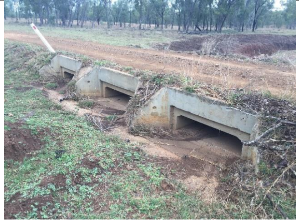
2. Downstream view pre-event condition, post event silt & debris.
