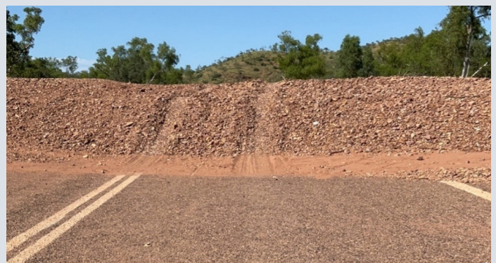
Gregory Downs–Camooweal Road – river gravel over road at Police Creek (March 2023)
