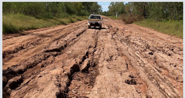
Gregory Downs–Camooweal Road – damage from Northern and Central Queensland Monsoon and Flooding (April 2023)
