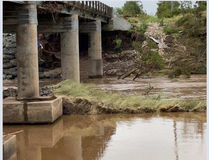
Lockyer Creek Bridge – abutment scouring (March 2022)
