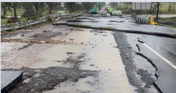
Gatton–Helidon Road – pavement damage (March 2022)
