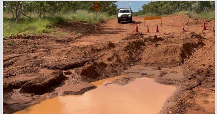
Gregory Downs–Camooweal Road – washouts following Northern and Central Queensland Monsoon and Flooding (February 2023)
