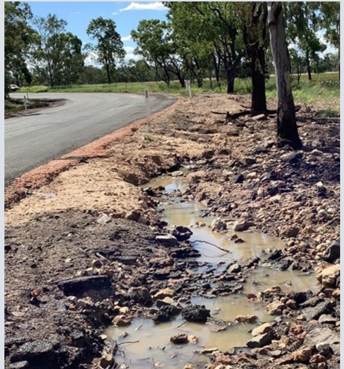
Toowoomba–Cecil Plains Road – shoulder scouring (March 2022)
