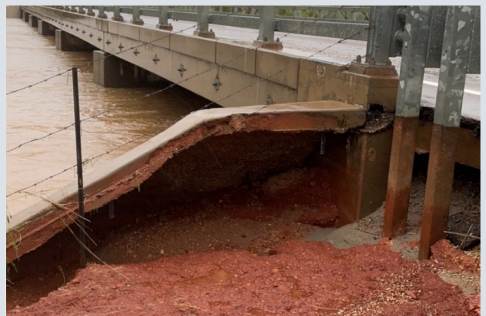
Barkly Highway (Mount Isa–Camooweal) at Inca Creek – damage from Northern and Central Queensland Monsoon and Flooding (March 2023)
