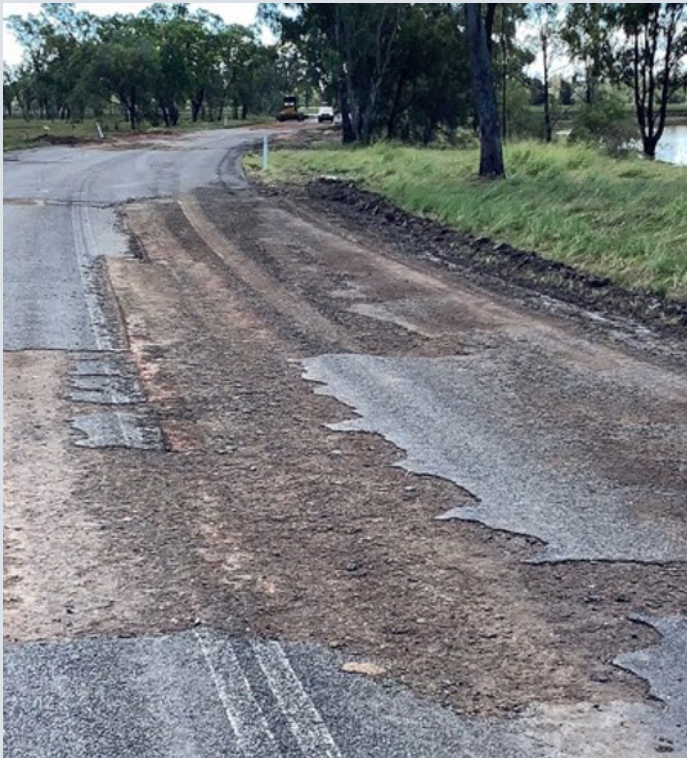
Toowoomba–Cecil Plains Road – seal delamination (March 2022)
