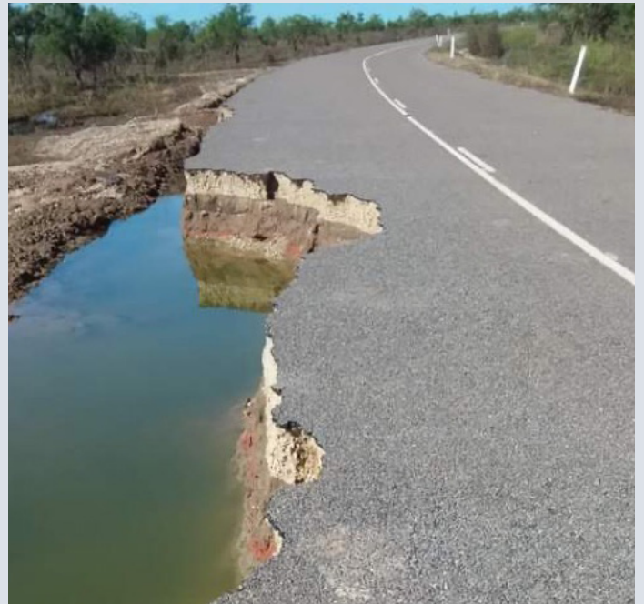
Wills Developmental Road (Julia Creek–Burketown) – damage from Northern and Central Queensland Monsoon and Flooding (March 2023)
