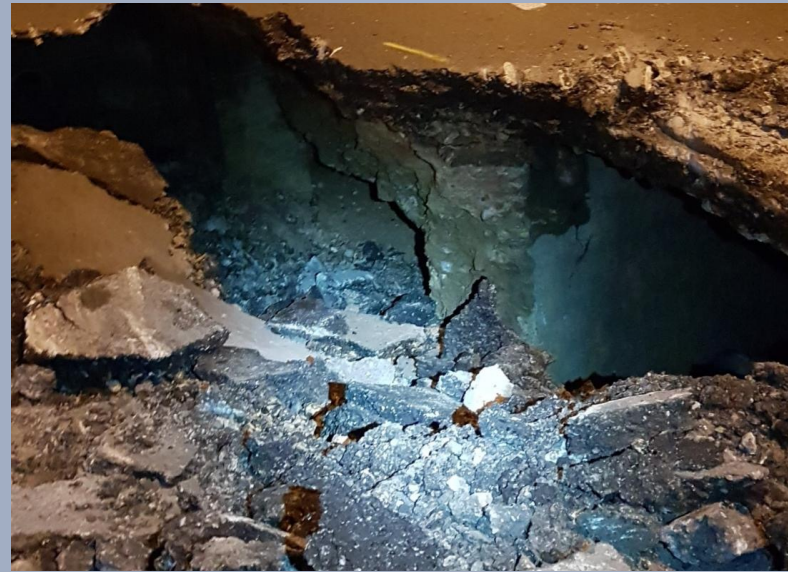
Image: Gympie Arterial Road – erosion under pavement (evening of 18 March 2022)
