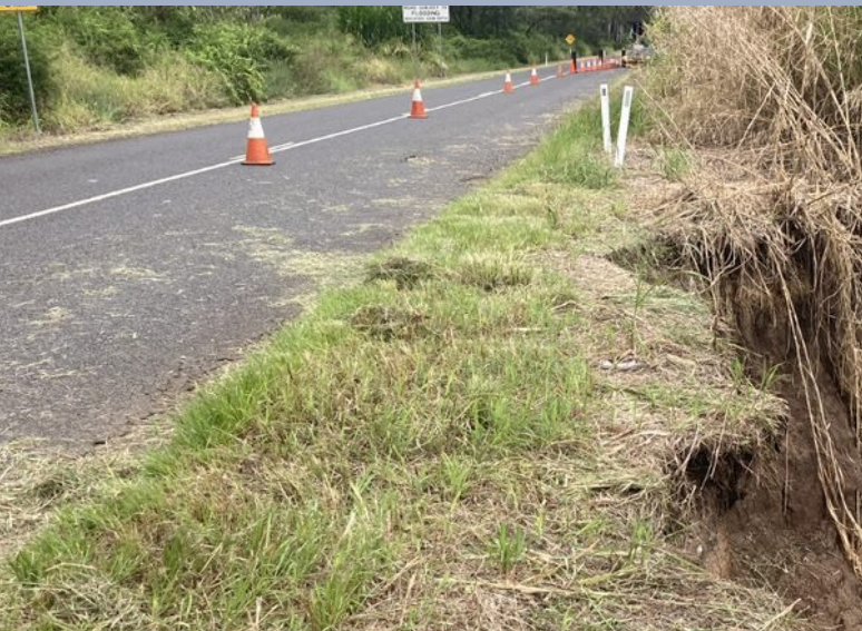
Image: Mulgowie Road – Laidley Creek scouring damage (February 2022).
