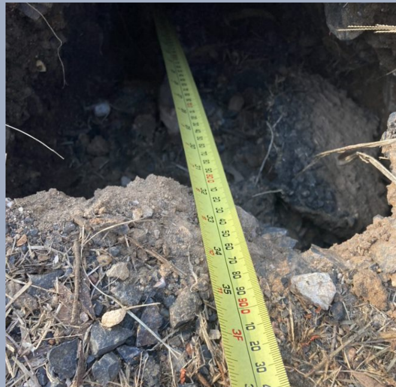
Image: Mulgowie Road – measuring pothole depths (February 2022).
