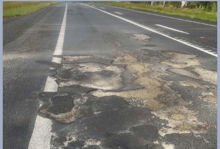
Image: Bruce Highway (Gin Gin–Benaraby). Pavement shoving north of Takilberan.
