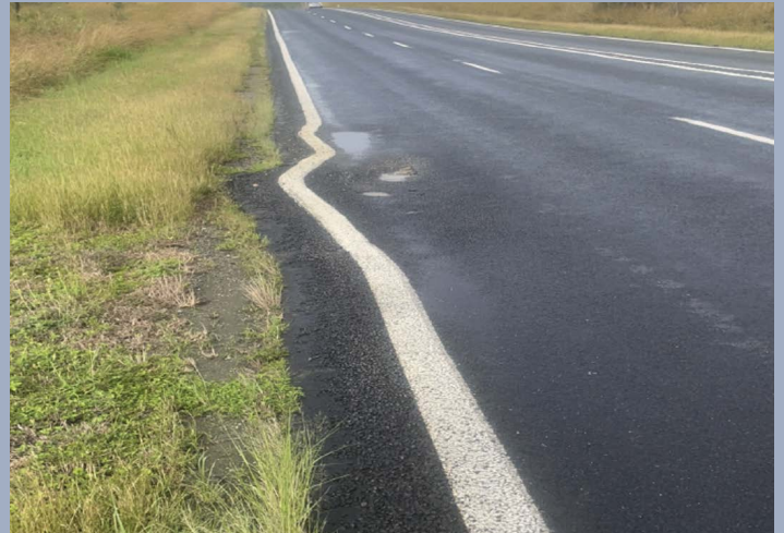
Image: Bruce Highway (Gin Gin–Benaraby). Pavement rutting south of Rosehill Road.
