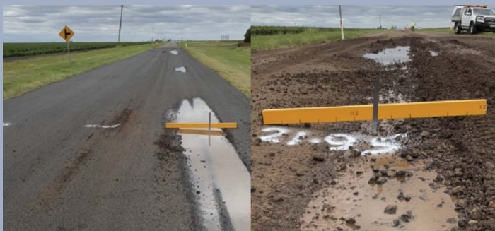
Images above: Bowenville–Norwin Road. Further damage after rain in late January 2022
