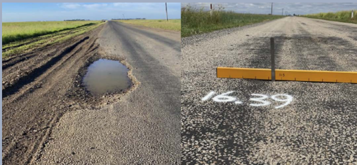
Images above: Bowenville–Norwin Road. Pothole after rain in December 2021 and subsequent repairs in January 2022.
