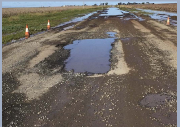
Image: Bowenville–Norwin Road. Significant damage to the road surface after combined weather events (May 2022).
